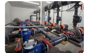
St. Kitts Bird Rock Desalination Plant 2,000,000 GPD
